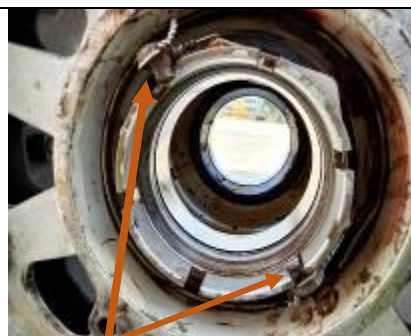
Figure-5: Upper part of the locking bolt attached with the locking wire of the wheel assembly
